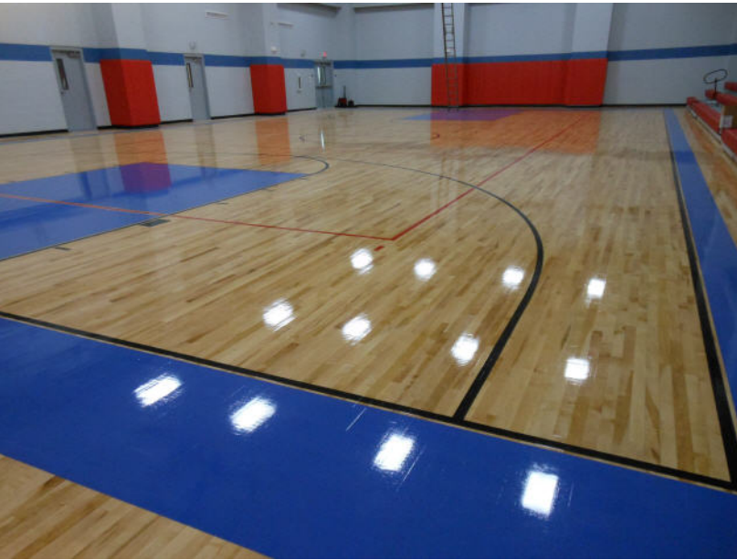
Sealing and finish issues
